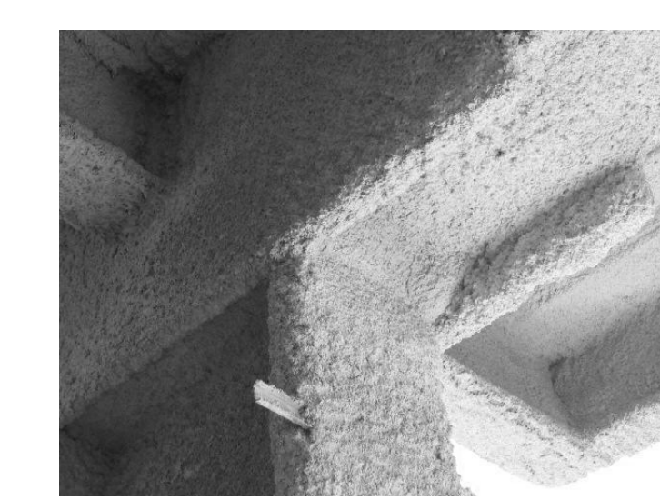
FIELD ERECTION GRAPHIC NO. 5B - FIREPROOFING ACROSS THE BOTTOM OF THE GAP
